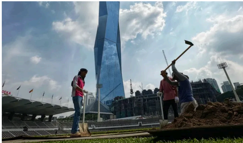
Workers meticulously restore the hallowed grounds of Stadium Merdeka. In the background, the towering Merdeka 118 symbolises Malaysia's progress, a striking contrast to the stadium's timeless charm. (Pix: Fernando Fong)
